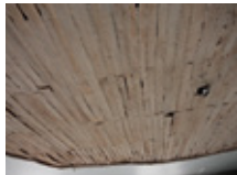
Area of fallen plaster.
